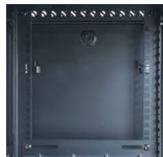
Vertical cable ladders Are used to attach cable and PDU (power distribution units)
